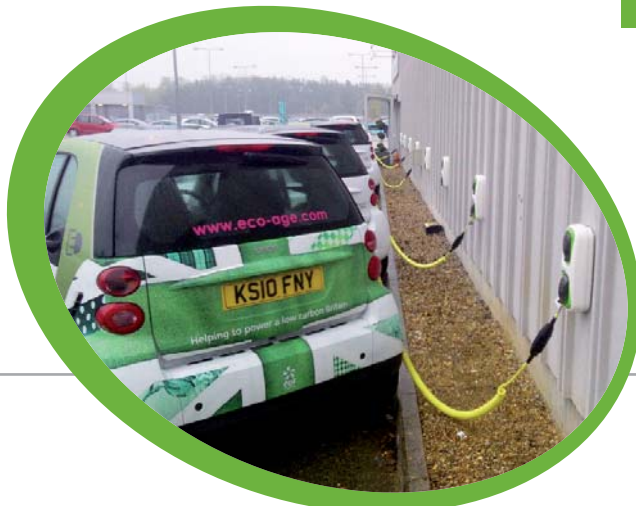
Commercial EV charging
